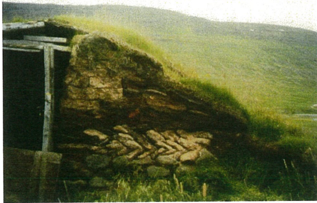
In the gable of the sheep barn at Hof in Hjaltadalur you can see milk-pen blocks that are lying flat, at the top, and set overlapping each other below. At the bottom of the wall are stones. The barn is roofed over with grass sod turf.
