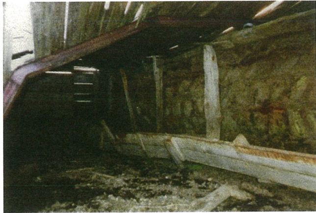
A cow-barn wall at Halldórsstaðir made out of clamped blocks and strips . The stalls were opposite this wall, and protected it. The far wall, to more than halfway up, was made of stone with strips between the courses.
