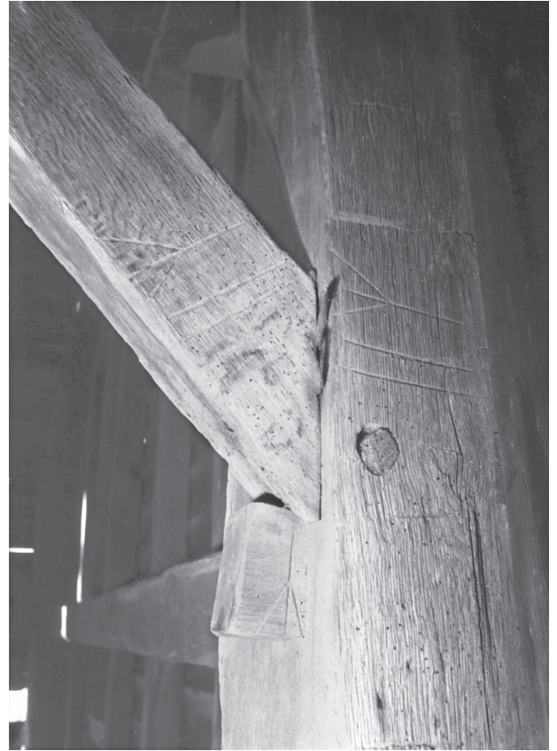
Scribe rule barn in Chatham, N.Y., with packing or distance piece driven to take up space needed to fit brace into made-up assembly of post and beam. Brace, post and packing piece are all marked for reassembly after scribing.
