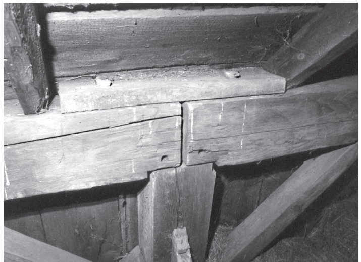
This strange arrangement in a barn in Rochester, Vermont, uses the post-top tenon as a sort of free tenon to join the plates, though pins are invisible. The builder must have realized the inherent weakness of the connection and added the fish plate on top, secured with two pins.
