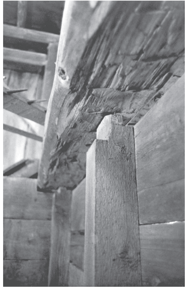
This partially withdrawn stud in a barn in Shaftsbury, Vermont, was relieved at its end to make its tenon barefaced. The relief cut was not angled as usual, and gives the appearance of a second cheek and shoulder.
