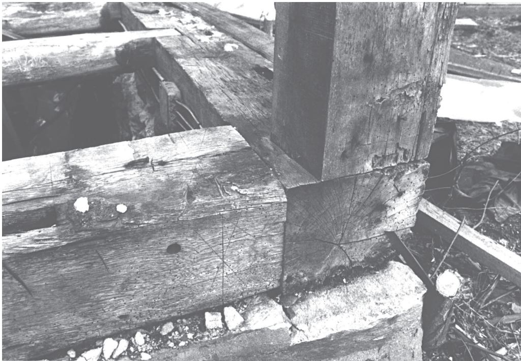
The typical blind sill corner joints on this house frame in Charlemont, Massachusetts, give little clue to their inner mortise and tenon configuration. The first joist to the rear, hewn flat only where necessary, joins the sill in a butt cog. Timber sills and girders, historically a natural part of the timber frame, have virtually disappeared from modern American work.
