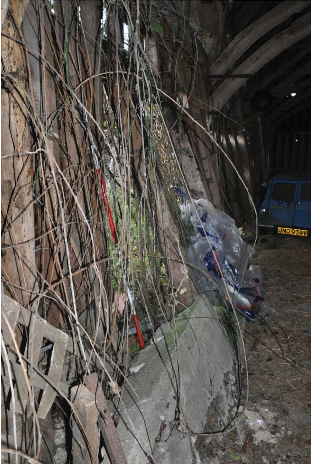
Bay 5 - Wall Frame Leaning to the East
